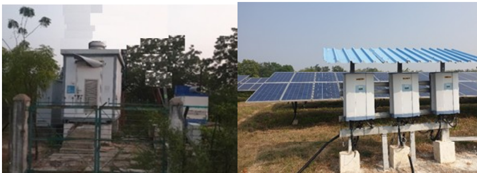
Solar Power Plant and Solar Panels installed on the University Buildings.
